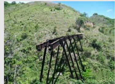
A bridge near Agua Caliente, Guatemala, shows evidence of large-scale metal theft earlier this month.
