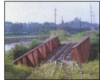
This damaged bridge, at Villa Canales, gives some idea of the scale of the task facing the RDC in reviving railways in Guatemala.
